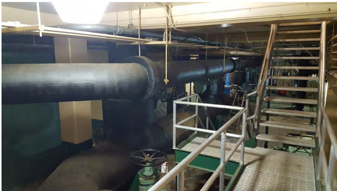
Photo #1: HAN 400 Tar Coating on Foam Pipe Insulation (ACM)
