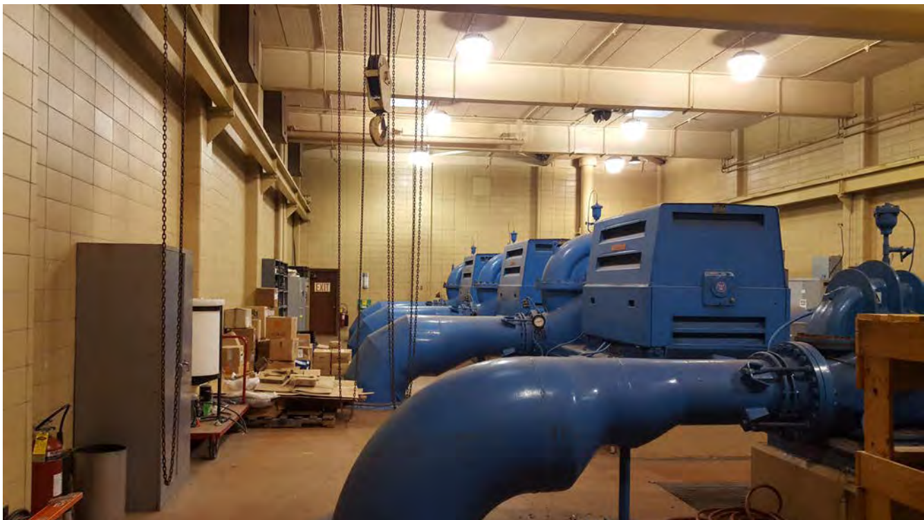
Photo #4: HAN 604 Pump Wiring (Assumed ACM)
