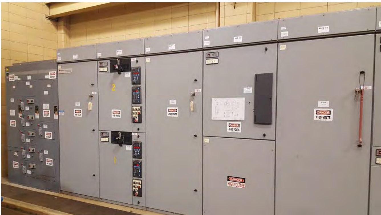
Photo #3: HAN 602 Pump Motor Control – Electrical Components (Assumed ACM)
