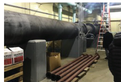
In order to increase the capacity of the Van de Water Treatment Plant, several modifications will need to be implemented including upgrades to treated water piping.
