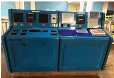
Filter controls will be upgraded to provide state-of-the-art, fully automated backwash sequencing.
