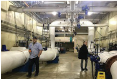
Filter Gallery: Filter-to-waste piping must be evaluated to confirm capabilities.
