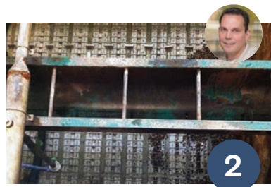
Southern Indiana Operations and Treatment Center Filter Media and Underdrain Rehabilitation Indiana American Water, IN
