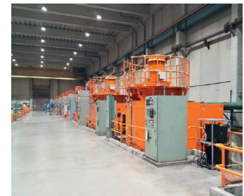
Lake Huron WTP Pumping Improvements Great Lakes Water Authority, Detroit, MI
